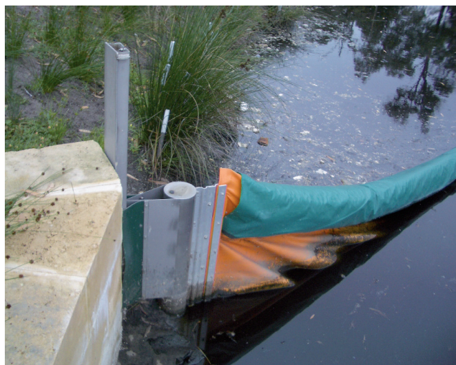
▲ Tidal compensator permanently installed.
