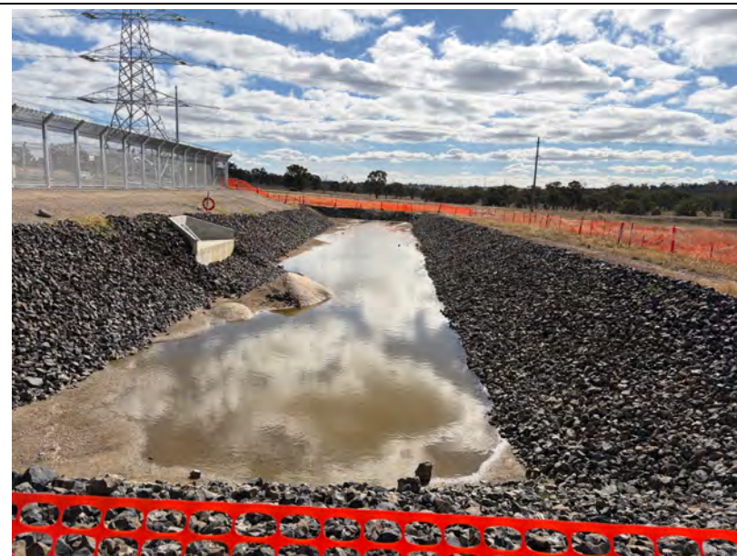
Transgrid Switching Station: Sediment basin operational for collection of stormwater, treatment and discharge/reuse of water onsite for dust suppression.
