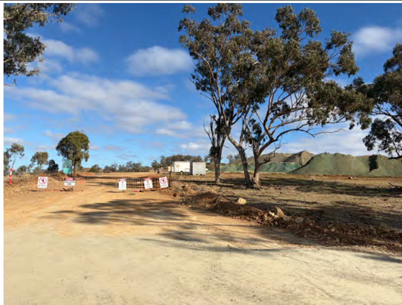
Naturally occurring asbestos area – exclusion zone in place with appropriate signage. Nacap reported that licenced asbestos hygienist in attendance and air monitoring ongoing. Regulatory notifications and community notifications in place. Stockpiles were observed to be stabilised with polymer.
