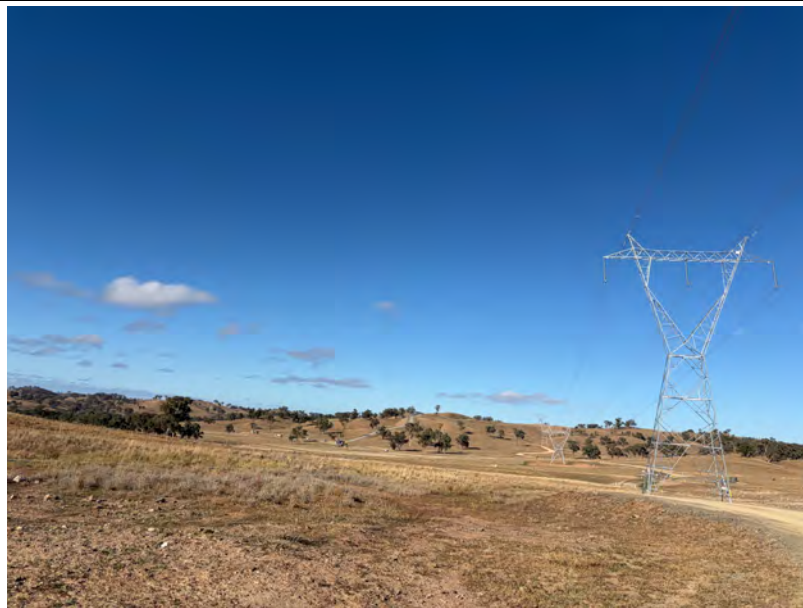
Transmission towers and power lines installed connecting substation and switching station
